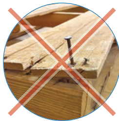
Raised nails greater than 1/8" are NOT ALLOWED .
